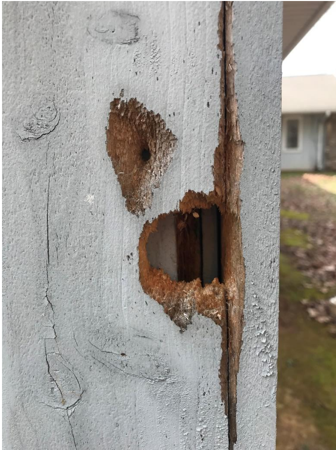
Fig. 3 – Deterioration of siding
