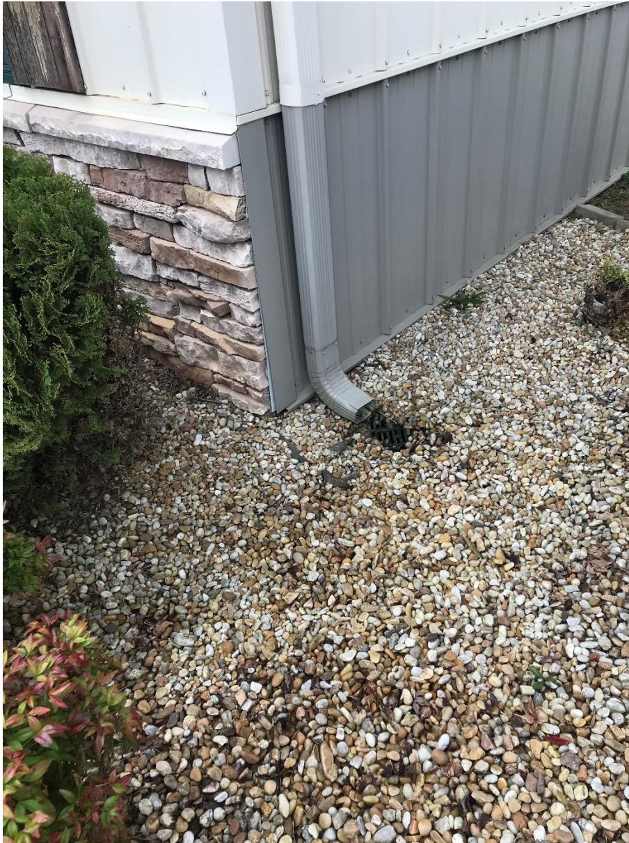
Fig. 2 – Downspout draining covered by dirt/ gravel
