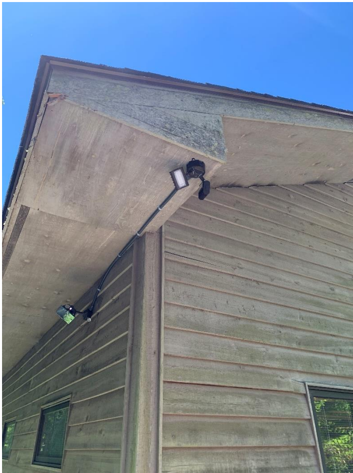
Fig. 2 – Deterioration of wood siding
