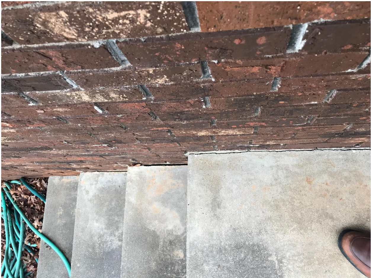
Fig. 2 – Crack along entry stair
