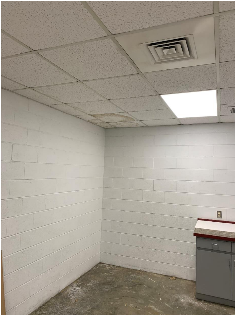
Fig. 2 – Leak above ceiling
