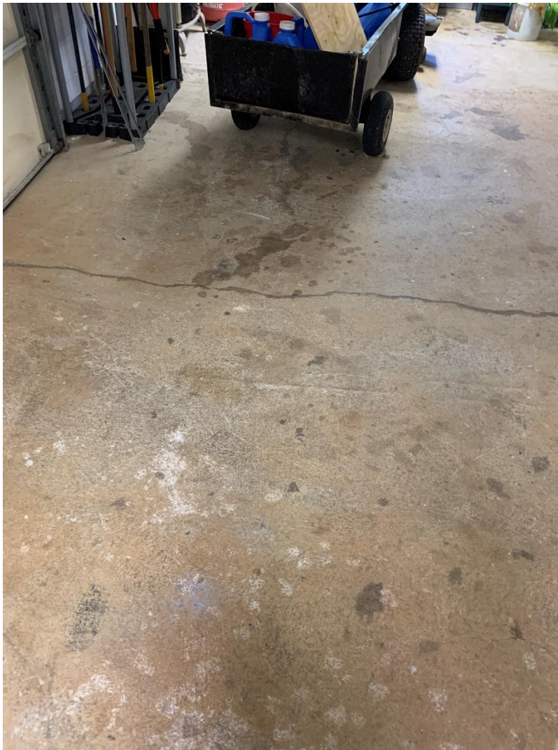
Fig. 2 – Crack in Slab on Grade
