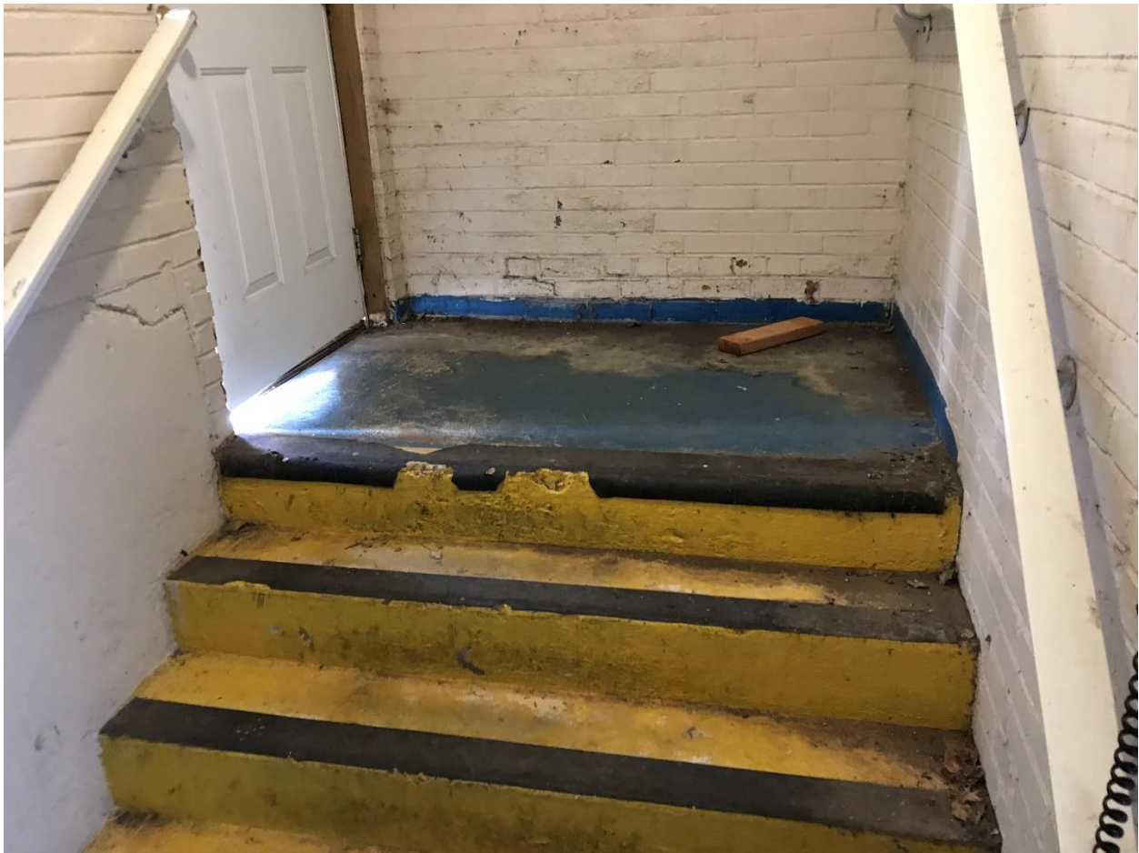
Fig. 2 – Deterioration of interior stair
