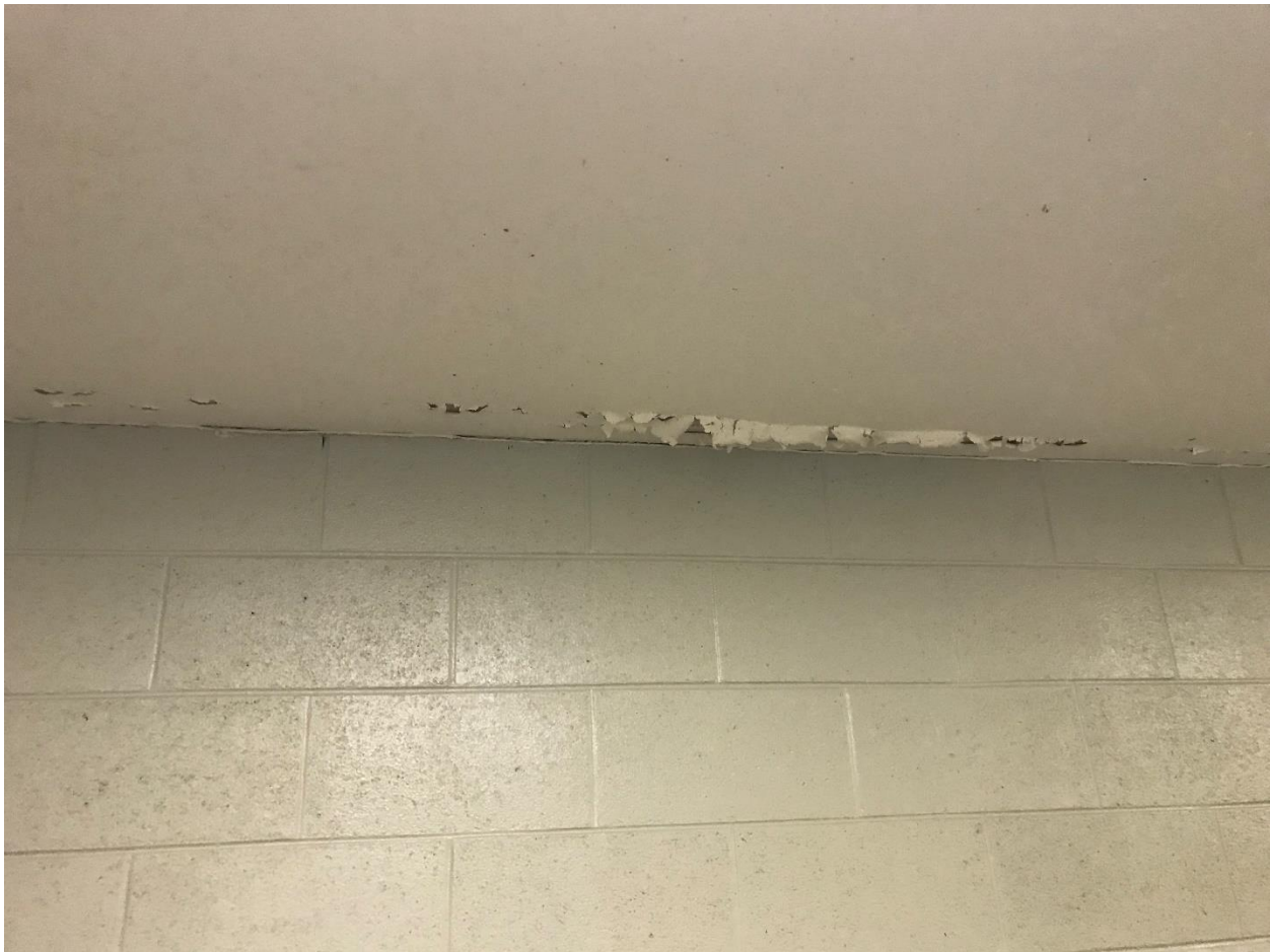
Fig. 1 – Gypsum ceiling peeling
