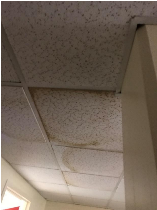
Fig. 2 – Ceiling damage from water intrusion.
