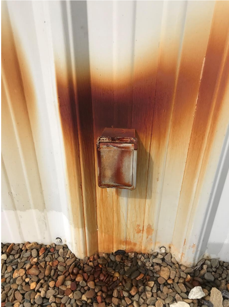
Fig. 2 – Exterior rust/ corrosion
